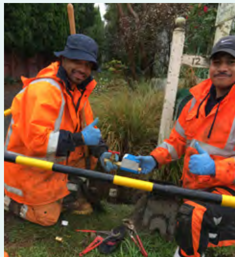
Installers Eru Te Kahika (left) and Lu Fonoti (right) with one of the 250 smart meters Wellington Water is putting in Greytown, Wairarapa.
